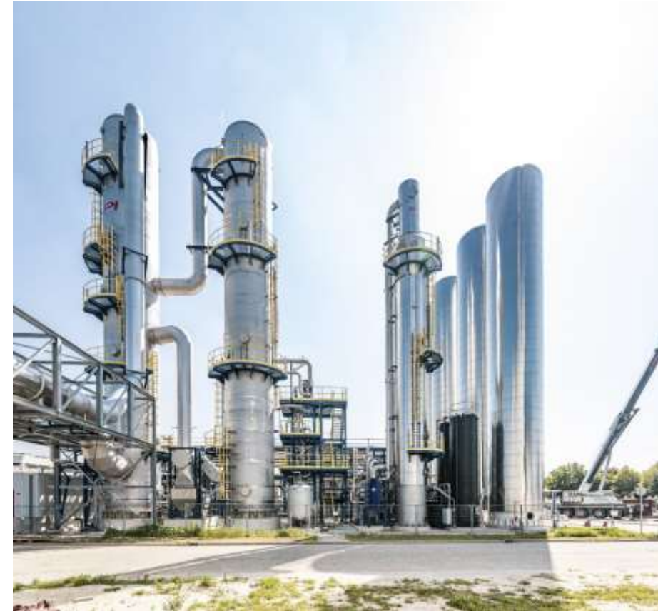
Source: Duiven plant with carbon capture unit, AVR.
