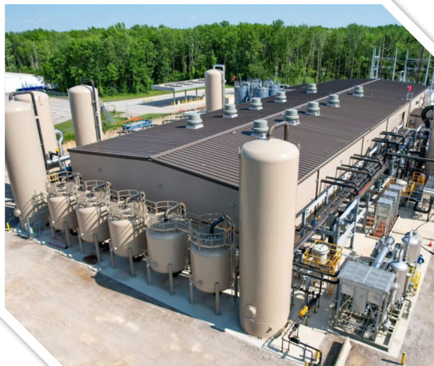
Lorain Renewable Natural Gas Facility
