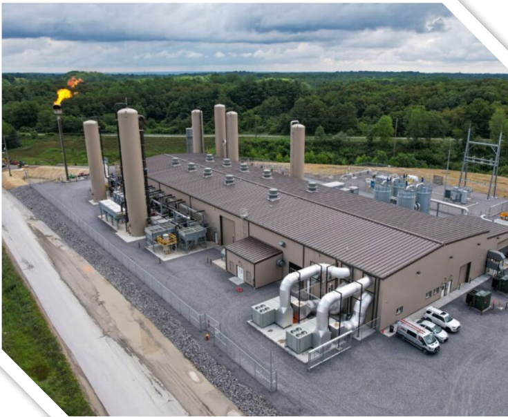
Limestone Renewable Natural Gas Facility
